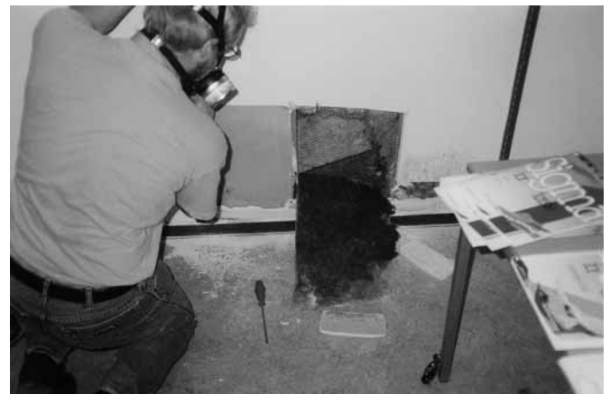
Fig. 5 Engineer working on a waterdamaged school detecting heavy mold infestation on the reverse side of the building material. Note the protection mask. Photo: Kristian Fog Nielsen
