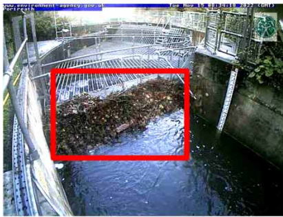
Image of a trash screen blocked with debris
