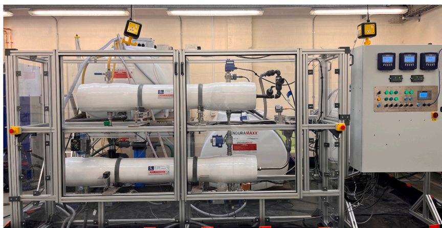
Fig. 2. The installed pilot scale 120-bar batch RO system at the University of Birmingham, UK, showing 8-in. RO module (top) and work exchanger (bottom) inside safety enclosure.
