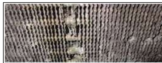
Figure 2: Fins corrosion and salts accumulation of outdoor heat exchanger
