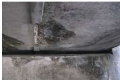
Figure. 3, span 2-Girder 1, concrete spalling, exposed tendons due to exposing fire.
