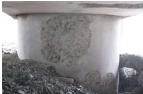
Figure. 6. Span 2-Girder-2 Pier concrete spalling due to exposing to fire.
