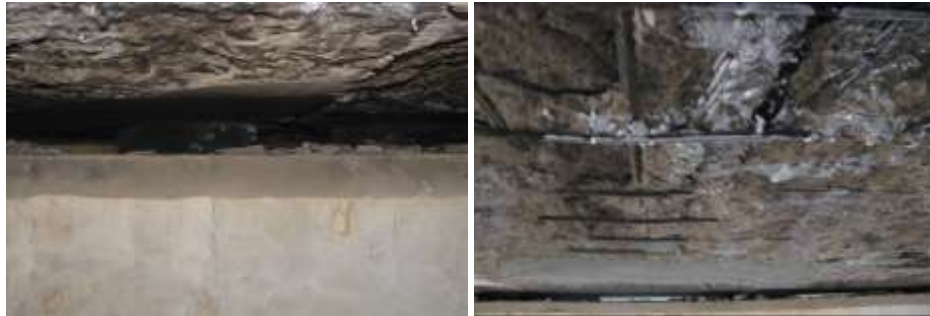
Figure. 5. Cover of right hand side a beam bearing after fire.
