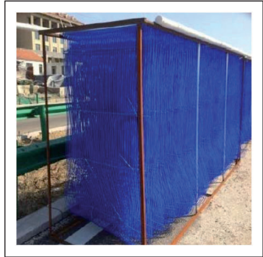
Figure 4. The capillary heat exchanger buried in the coastal area.
