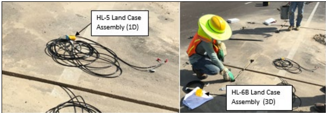
Figure 4: Installation of HG-6 Geophones in (a) HL-5 Land Case (1D) and (b) HL-6B Land Case (3D) Assemblies
