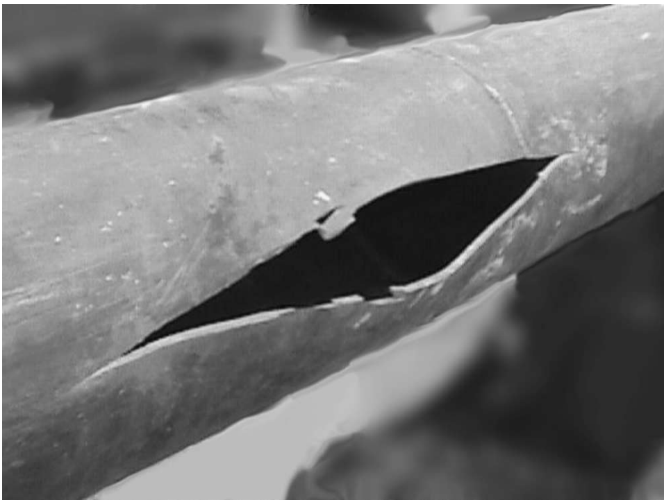
Fig. 1. Visual aspect of the SCC failure in a 14 inch ERW oil pipeline. (Failure case 1.)
