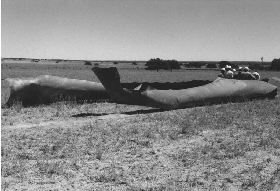
Fig. 5. Failure in a natural gas pipeline, 23 km downstream from the closest compressor station. (Failure case 3.)
