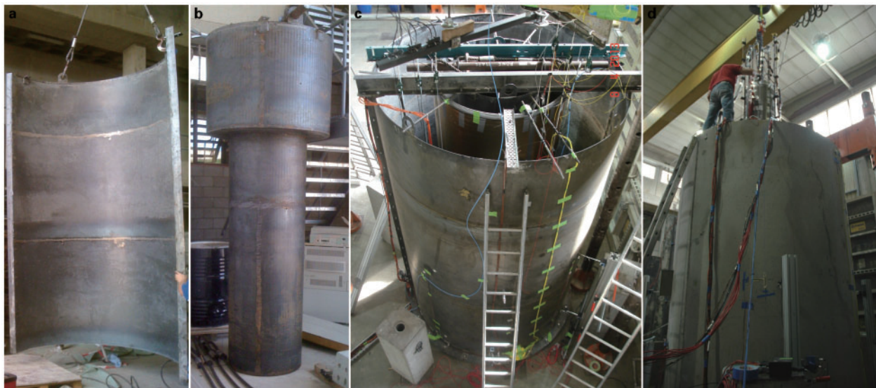
a one of two steel cylindrical segments of outer mould ( \varnothing \sim 2.1 m; height \sim 3.5 m); b inner steel tapered mould ( \varnothing \sim 0.5 m); c assembled mould before casting of concrete buffer; d cured concrete buffer during installation of heater
