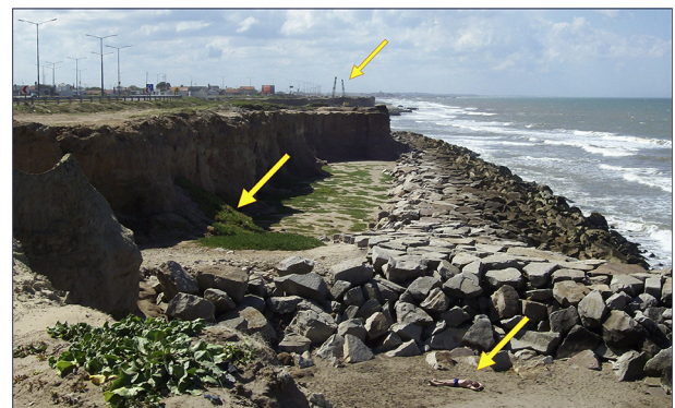
Fig. 9. Santa Helena's coast in 2011. The restricted backshore is dominated by vegetation and partially covered by mixed ramps. Notice the mound's dimensions in comparison with the man below, how close is the road from the cliff and see how the heavy machineries are working on mounds at the background. See the location of this photograph in Fig. 4 ("C").
