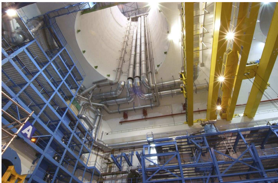
Figure 9.5: Air ducts installed for ventilation in the shaft and main cavern.
