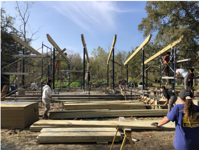
Figure2: Students working on the construction of the outdoor teaching space at Sugar Roots Farm (lifting beams with a material crank lift) (Small Center).
