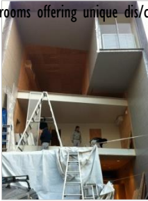
Figure 17: View to share house cube cavity during construction process: Floor slabs and one of four fourth floating box inhabited with seventh room volume; [Hirano, 2012]
