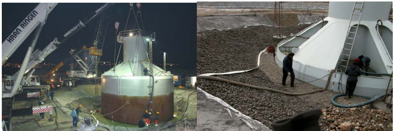
Figure 3: Installation of the prototype in Frederikshavn by suction. a) before installation. b) after installation .
