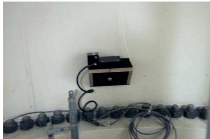
Figure 10. Accelerometer mount at the connection between the tower and the foundation.
