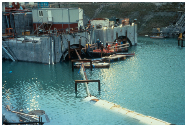
Fig. 15: Inundated tunnels and ramp on Sprogø
