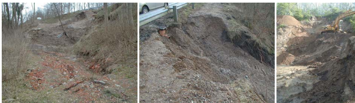
Figure 4. (a) Slide failure blocking private road; (b) The missing bicycle lane; (c) The hunt for Tertiary clay floes
