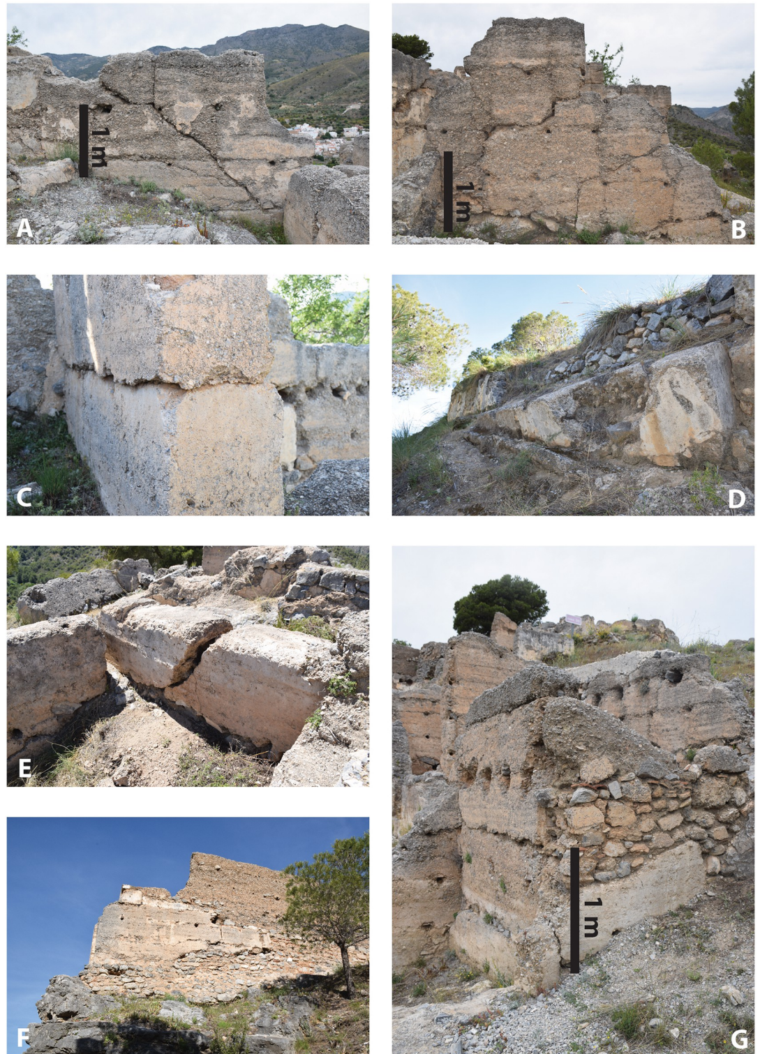
Fig 2. Examples of seismic damage and restoration observed at El Castillojo: A-B: shear cracks in Building 4; C: horizontally-shifted block of rammed earth in Building 3; D: tilted block of the outer wall; E: broken and displaced wall in Building 30; F: post-earthquake restoration of the western gatehouse and G: Building 10. Photographs by P. Forlin.
