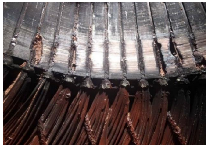
Fig 2 Damage on surface of a stator core due to rotor-stator rub
