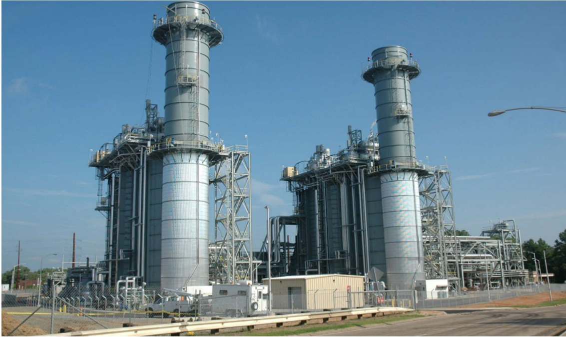
Figure 2-12 Natural gas-fired power plant (PowerGrid International, 2016)
