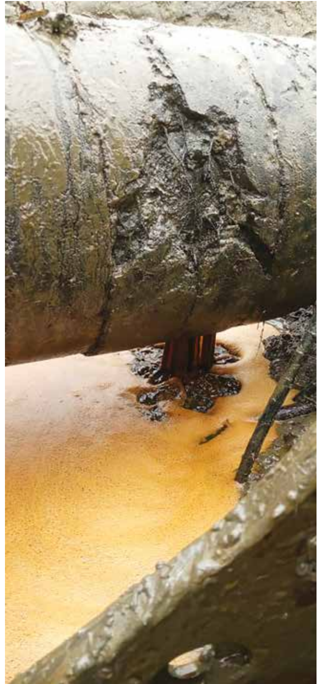
A pipeline leading to an oil spill and pollution on an Agip site in Ogboinbiri.
