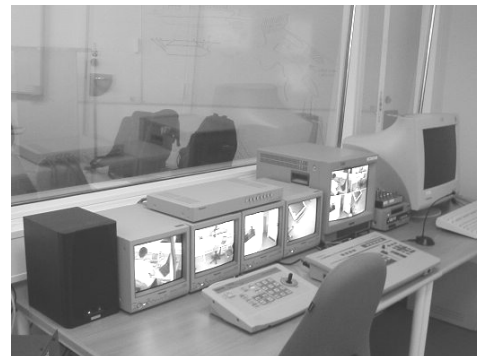
Figure 10. The control room
