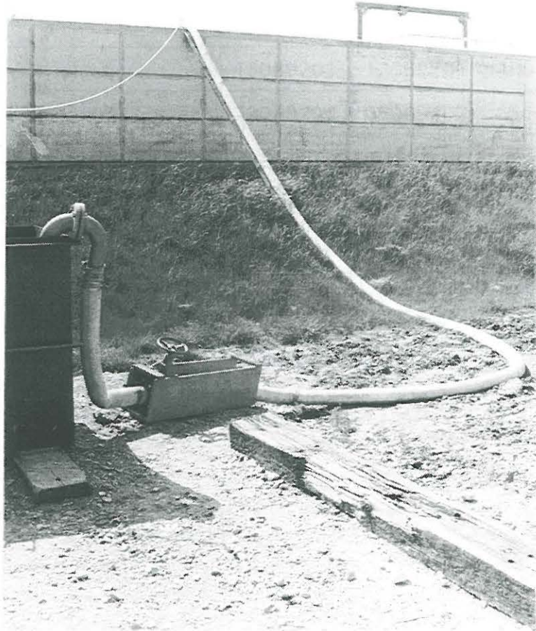
Fig. 6.5. Outlet flow pump system.
