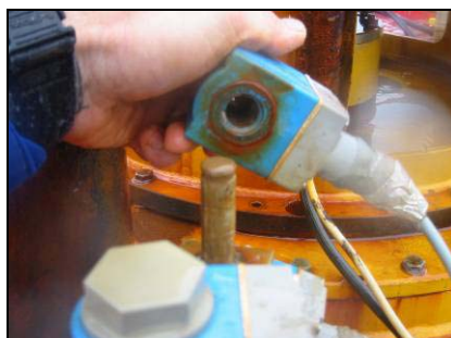
Fig. 4.4 Saltwater corrosion of solenoid (23.06.03)
