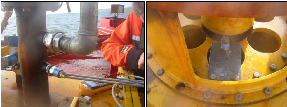
Fig. 4.1 Aeration tube water level switch installation and siphon turbine water level switch.
