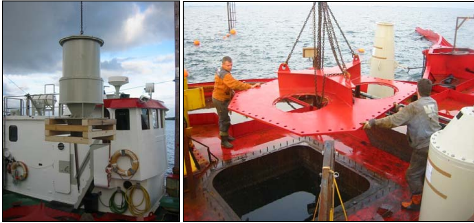
Fig. 4.11 Unloading of turbine centre and installation of floor plates section (runner & guide vanes)
