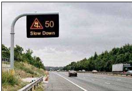
Figure 3: One of 36 MS4 signs on the M4 between J12 and J14 as part of the Highways Agency's On-Road MS4 Trial (source: The Highways Agency)
