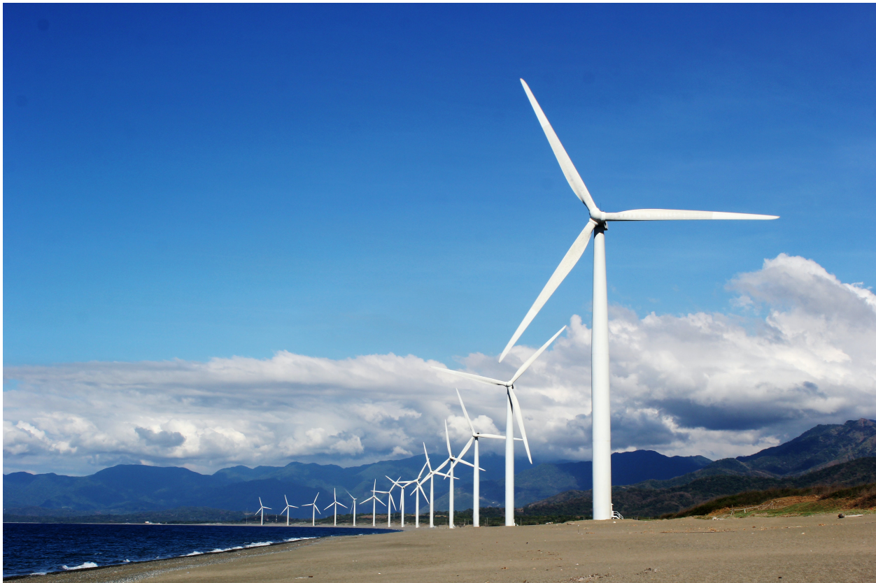
Figure 1.1: Wind turbine farm [37]
