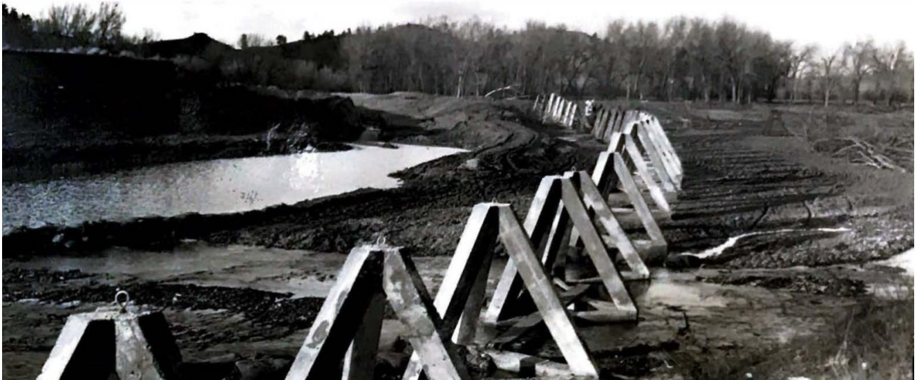
Figure 18. "Looking downstream at the back side of the row of tetrahedrons before placing the cables." Walter G. Attwell, Final Construction Report on Protection of Devils Tower Bridge, and Revetment Work on Belle Fourche River, November 25, 1930. (Courtesy NPS).
