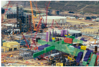
Fig. 11. Optimised crane planning and configuration for a modular project in Alberta, Canada [62].
