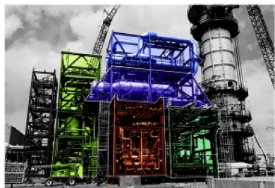
Fig. 3. – Modular process plant [26].
