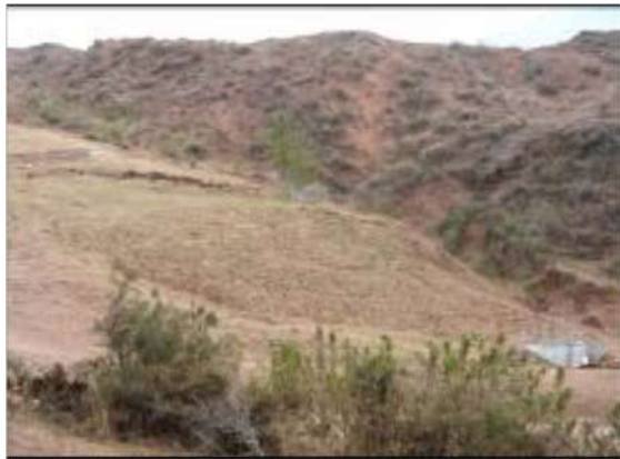
Fig. 23. Photograph of the slope rupture confirmed by site inspection, which was detected by DSS on a Peruvian LNG pipeline [158], [159], [167].
