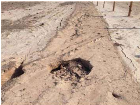
Fig. 17. Photograph of the eroded surface which caused the water infiltration event in Fig. 16 [160].
