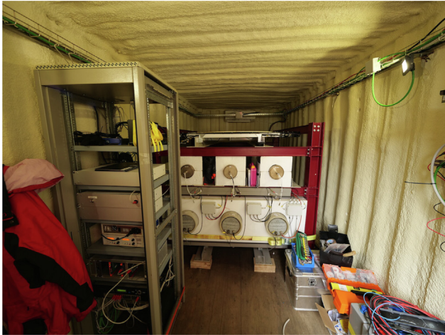
Fig. 2. MazORCA interior. The control and communications electronics cabinet is in the front, and the structure with ORCA’s detectors is in the back.
