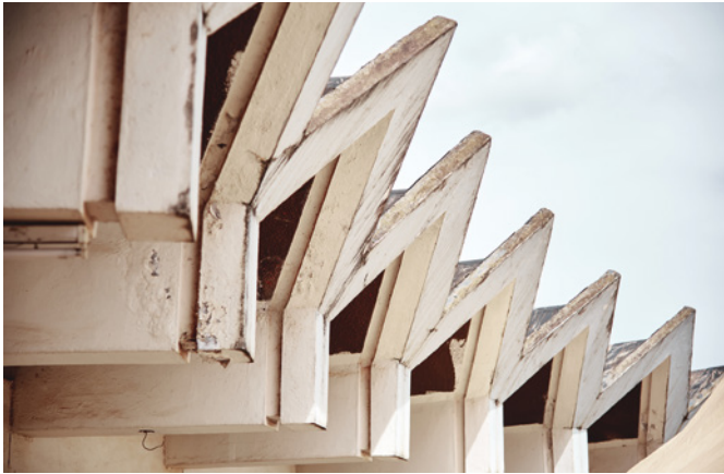
24 Roof details of the School of Fine Art and Industrial Design, Kyambogo University, Kampala, Uganda. © Timothy Latim, 2022.
