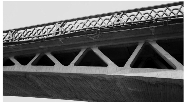
Figure 9. Detail of original railings and a concrete section of 6x6cm intact after 100 years. What a lesson!
