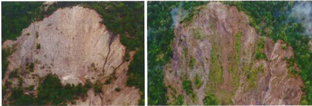
Figure 3: Photographs of the Sennindani landslide in 2015 (left) and 2022 (right) (Source: Forest Management Bureau, Chugoku Forestry Agency)
