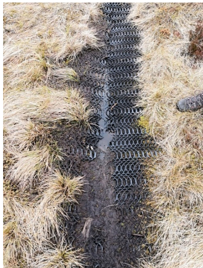
FIGURE 5 Area of failed track in a rutted section.
