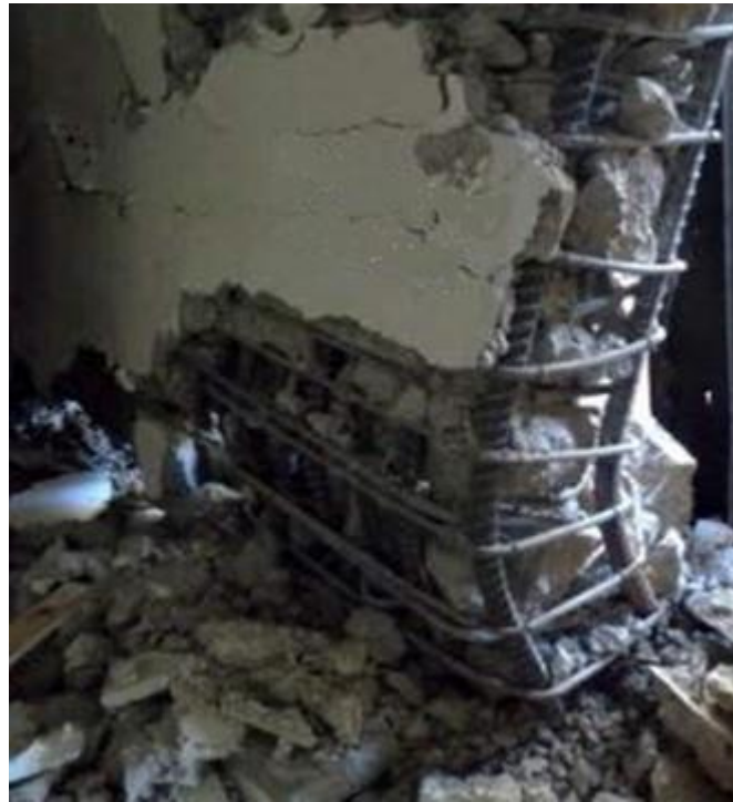
Figure 10. Out-of-plane induced damage in an RC wall after the New Zealand earthquake: Source: Sritharan et al.(2011)
