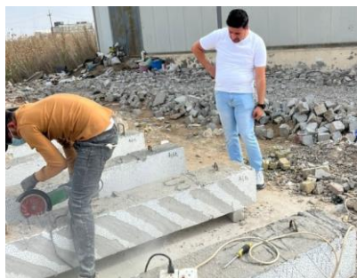
Figure 11. removed surface packers with the use of a grinding machine for carrying out the CFRP sheet
