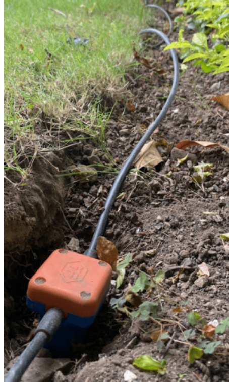
Figure 2: Seismo Seismic Detector (Source: RBtec Perimeter Security Systems)
