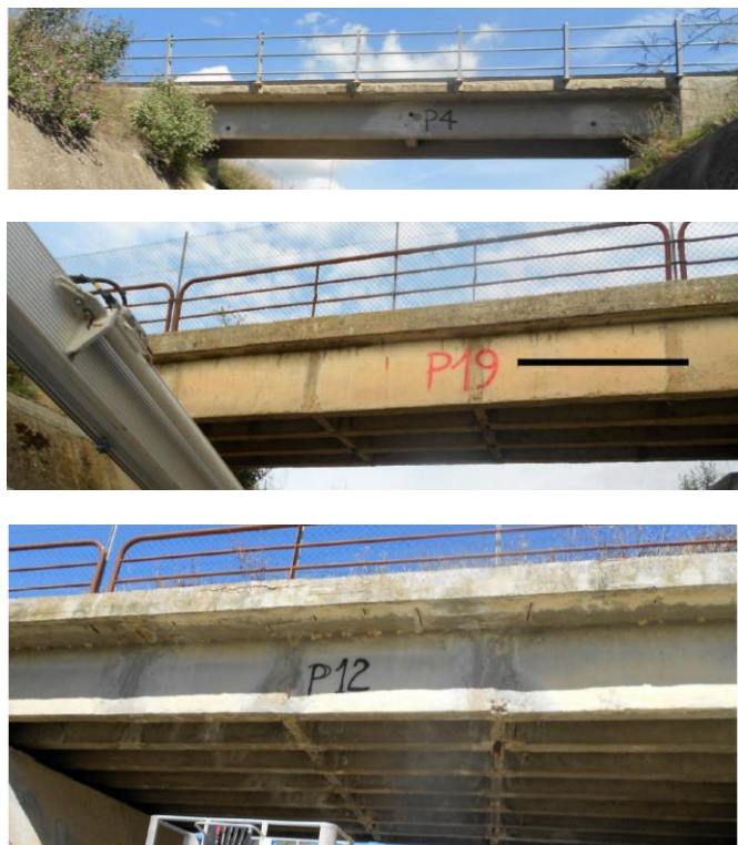
Figure 2 T1 type bridge (up), T2 type bridge (middle), T3 type bridge (bottom).
