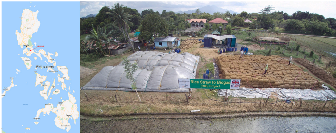
Fig. 1. R2B pilot facility in San Francisco, Laguna, Philippines. The picture shows the two 500 m 3 digesters (Left: digester covered with grey canvas and digesting rice straw. Right: preparation of digester with rice straw bales).
