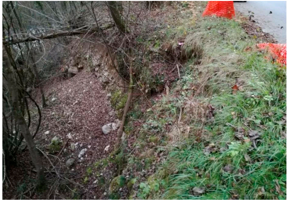
Figure 3. Landslide photograph code 025021_01c.
