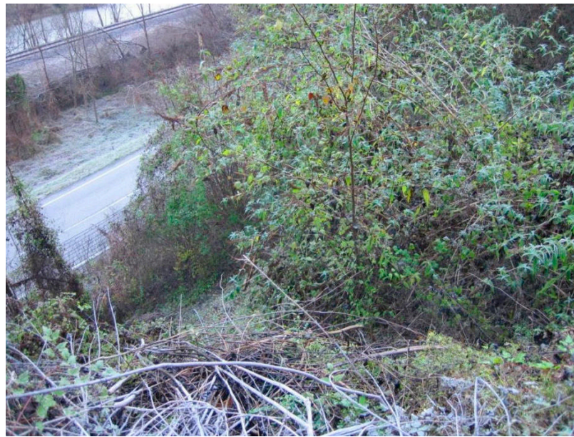
Figure 11. Landslide photograph code 025021_08c.
