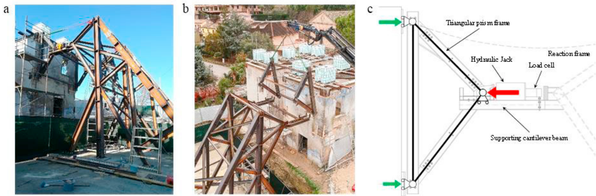
Fig. 3. (a) Pushing system during the test; (b) Assembly of the triangular steel frame; (c) Static scheme of the triangular steel frame.
