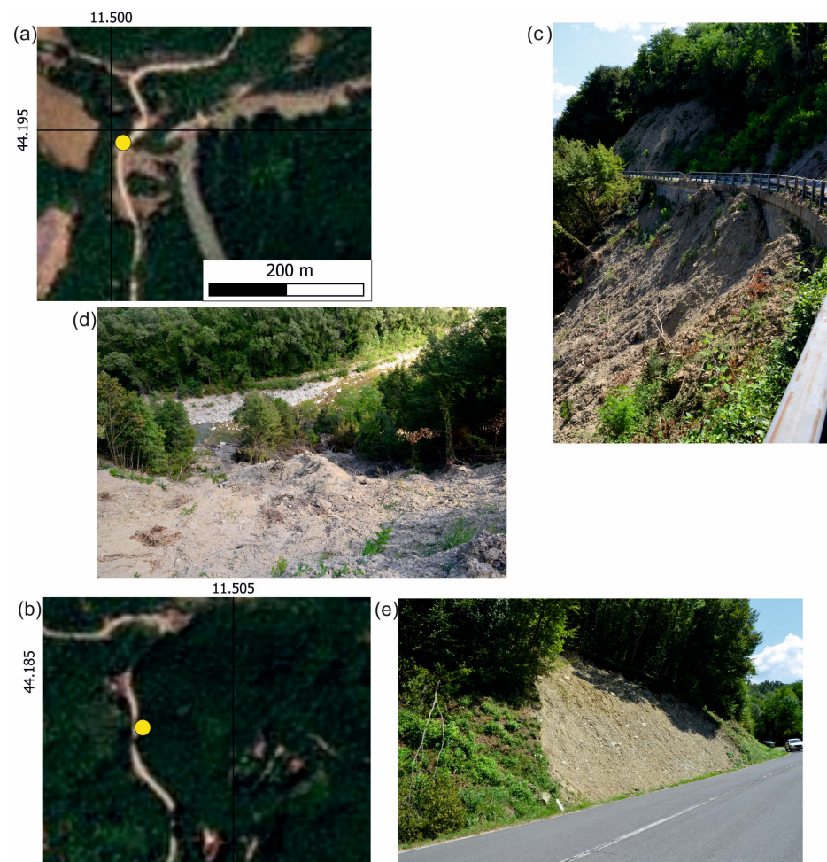
Figure 13. Satellite images and field photographs of landslides impacting the road network along Province Road SP610 in the Castel del Rio Municipality: (a,b) Planet images acquired on 23 May, yellow dots are the locations where pictures were taken; (c,d) field photos of a landslide impacting the road, the deposit area lies in proximity of Santerno River; and (e) field photo of a smaller landslide, not recognizable on satellite imagery. All the photographs were shot by M. F. Ferrario on 30 July 2023.
