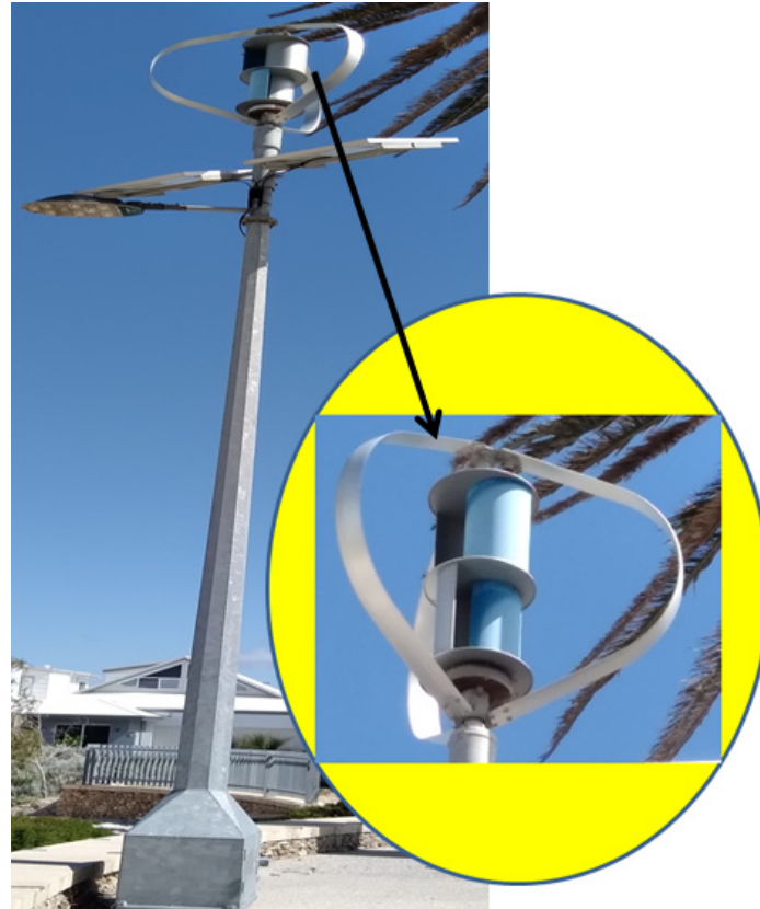
Figure 9. A miniature version of a wind turbine installed together with conventional PV panels to power the streetlight.
