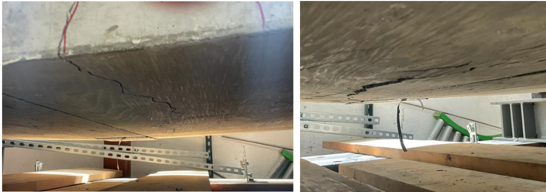
Figure 7.9: Cracks extending underneath specimen 1
