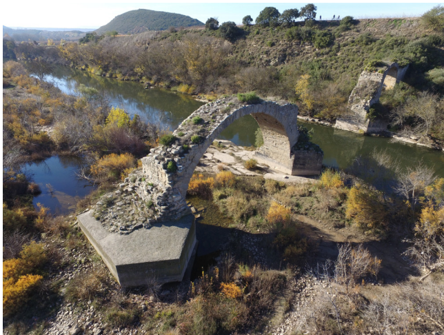
Figure 1. Upstream view of the remains of the bridge from a picture taken with a drone in 2017. The arch in the front corresponds to number 3 and the one at the back is numbered as 1.
