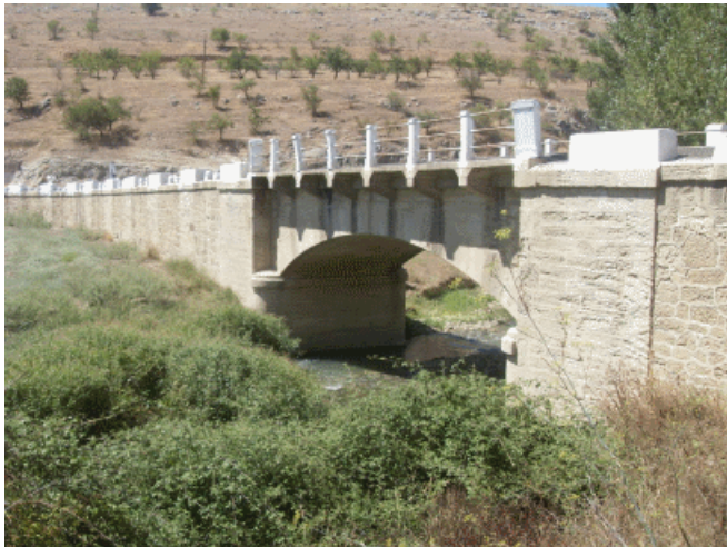
Figure 10: Bridge over the Alhama River (Granada), on the Secondary Road from Armilla to Alhama de Granada. Last Quarter of the 19 th Century
