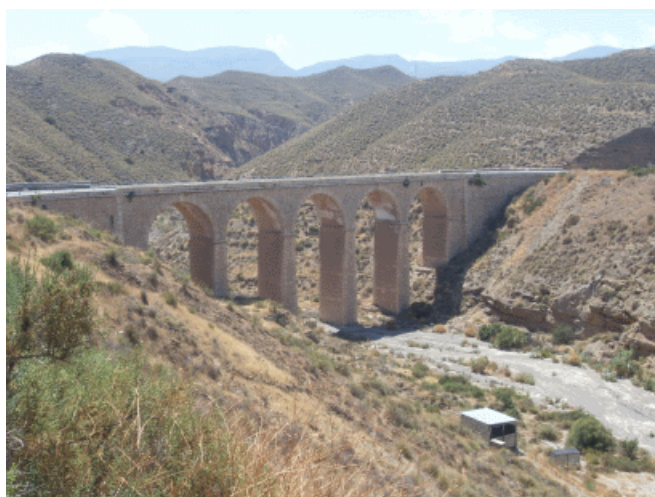
Figure 15: Rambla de Huéchar Viaduct (Almería), with five 14-m-span Arches over Sloped Piers 30 m High, on the Primary Road from Las Correderas to Almería. Third Quarter of the 19 th Century
