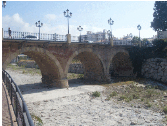
Figure 12: Bridge over Chillar River in Nerja (Málaga), with three Arches of 16 m in Spans, on the Secondary Road from Málaga to Almería. Last Quarter of the 19 th Century
