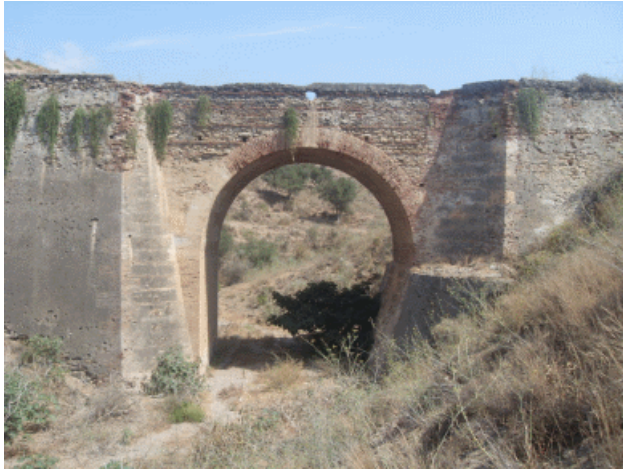
Figure 3: Jaral Bridge on the Road from Malaga to Vélez, with a Brick Arch of 11 Meters of Span, and with Tympana an Abutments of Rough Stonework, 1789. Domingo Belesta and Diego de Córdoba y Pacheco were the Military Engineers
