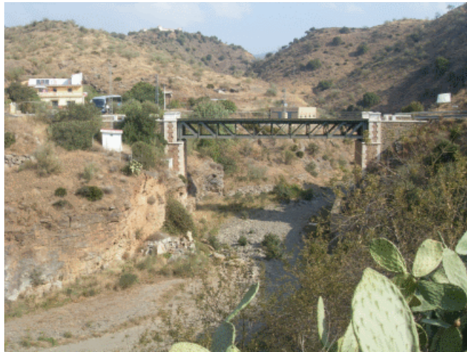
Figure 20: Bridge over the Campanillas River, with Triangulated Metal Beams on a Single Stretch with a 30-m Span, on the Road from Málaga to Almogía (Province de Málaga). At the End of the 19 th Century
