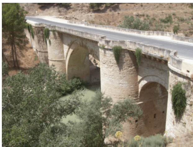
Figure 2: Bridge of Benamejí over the Genil River (16 th Century). Currently in Service as Part of the Secondary Road
