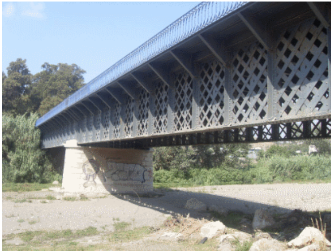
Figure 19: Bridge over the Vélez River in Torredelmar (Malaga) with a Straight Beam having Five 20-m spans, on the Road from Malaga to Almería, Towards 1865
