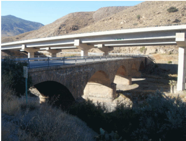
Figure 28: Bridge over the Nacimiento River in Abila (Almería) with Five Arches of 18-m Spans, on the Primary Road from Estación de Vilches to Almería, 1868. Juan Ezcurdia, Civil Engineer. Currently Reused as a Branch of the Exit for Freeway A-92
