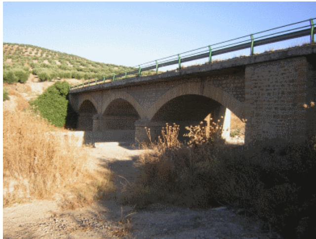
Figure 11: Bridge over Arroyo Salado Stream in Porcuna (Jaén), on the Secondary Road from Torredonjimeno to El Carpio by way of Bujalance. Last Quarter of the 19 th Century
