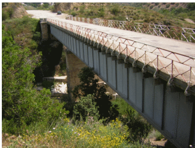
Figure 18: Bridge over the Víboras River in Martos (Jaén), with a Straight Beam with Two 30-m Spans, on the Secondary Road from Alcaudete to Granada by way of Alcalá la Real, 1863. Lucio del Valle, Víctor Martí, and Ángel Mayo, Civil Engineers
