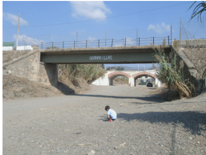
Figure 23: Bridge over Granadillas Stream in Benagalbón (Malaga), with a Straight Beam of Steel-Reinforced Concrete of Transversal Section p of a 15-m Span, 1920-30
