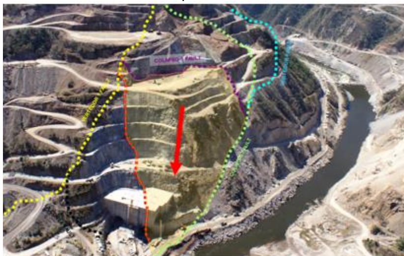
Figure 3. Block in unstable left margin faults delimited Collapse, Collapse 1 Collapse 2 and the granitic dike entrance portal diversion tunnels
