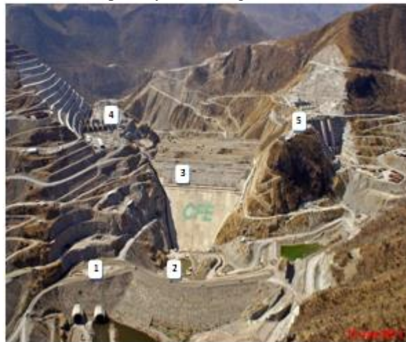
Figure 2. General layout of the project: 1, Diversion Tunnels, 2, Upstream Cofferdam, 3, Dam, 4, Open Channel Spillway, 5, Underground Powerhouse
