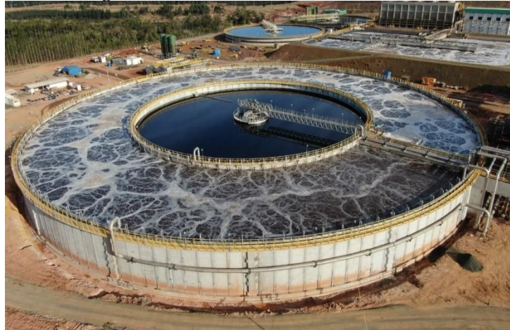
Figure 6- Effluent Treatment Station – ETS
