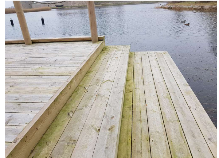
Figure 25: Signs of changing humidity in wooden decks.
