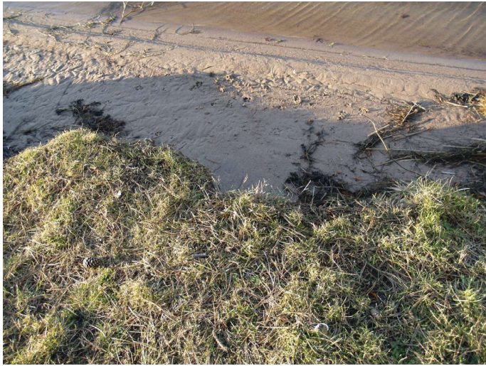
Figure 23: Signs of erosion in soft shoreline. © Vilborg Thorildsdottir
