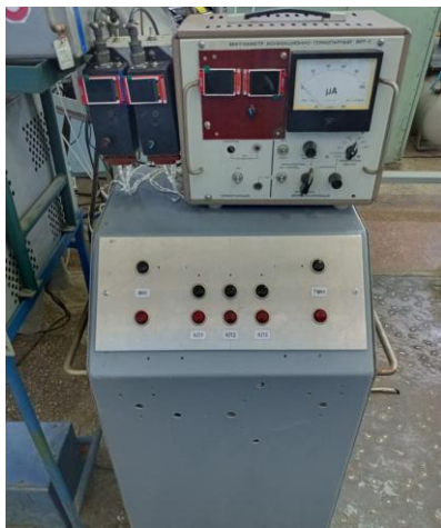
Fig. 5. Controlling unit of vacuum system
