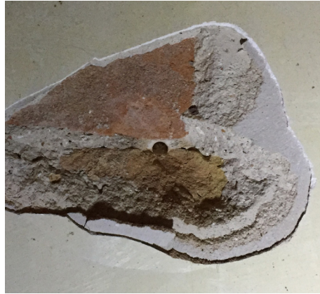
Perforación del revoco (RF5) Plaster perforation (RF5)
