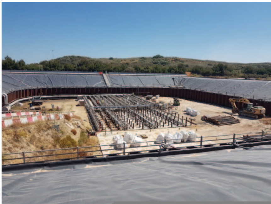
Fig. 6. – Area “Vasca A zone 2” (ISPRA/ARPA/Eni inspection photo of May 2019)
